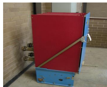
Ash Pond 6.6KV Circuit Breaker (CB) – AGL LY Magrini CB, Yallourn have a retrofitted Siemens CB as a replacement to the Magrini
