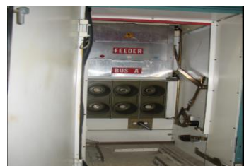
Ash Pond 6.6KV CB cubicle with Bus and Cable shutters open – similar Magrini bus work as the Yallourn switchgear
