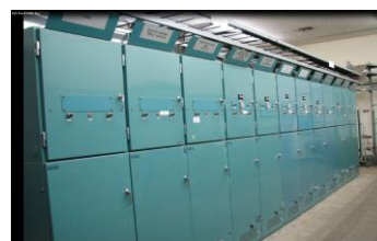
Ash Pond 6.6KV Bus – similar Magrini bus work as the Yallourn switchgear
